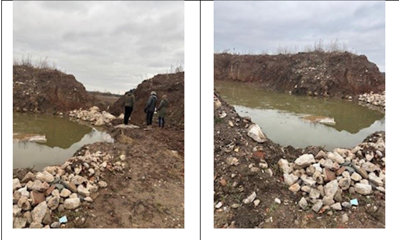
Berms located along the east side of the site and uncompleted stormwater works.
