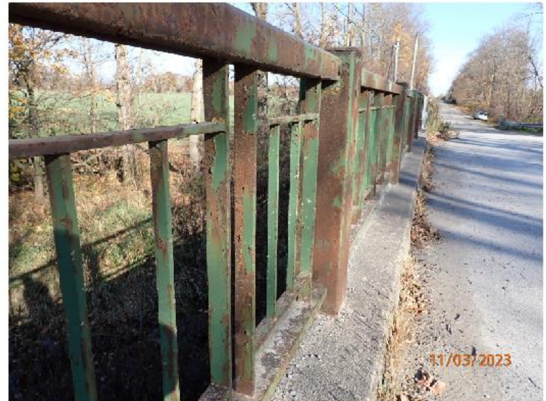
Photograph No. 4: 0418: Corrosion in railing (typ).
